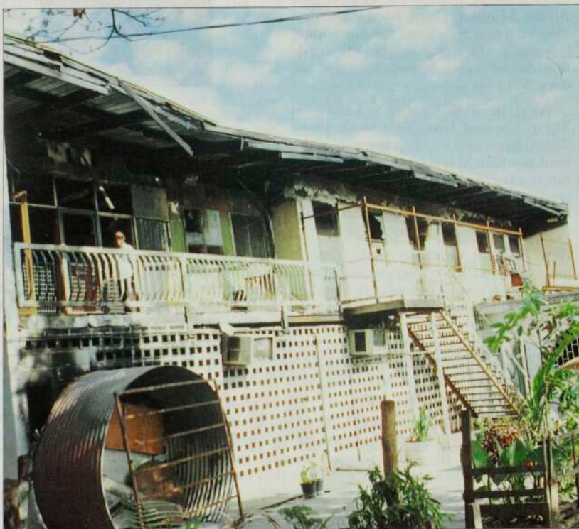
Wanton destruction: a nightclub destroyed by fire
