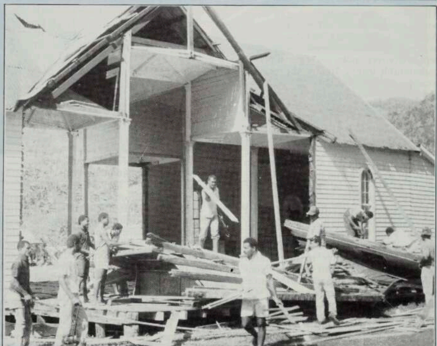
Faith: clearing out a damaged church
