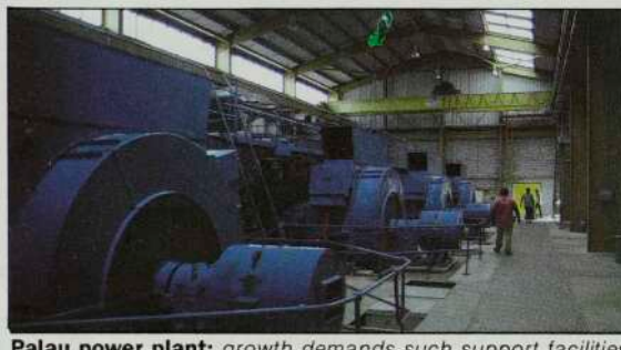
Palau power plant: growth demands such support facilities
