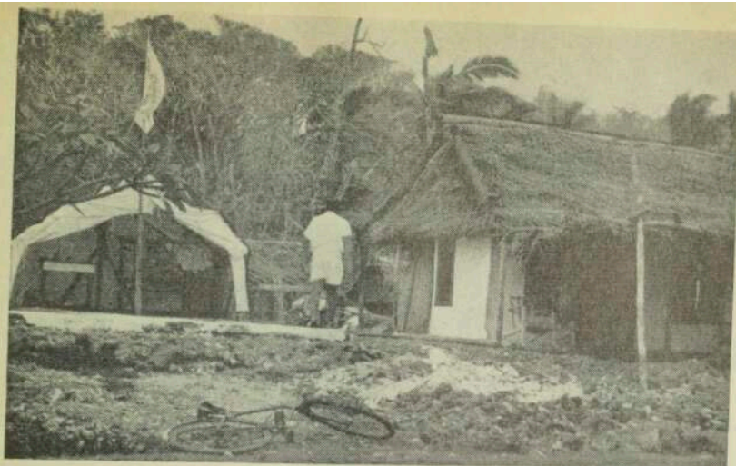
The house at the right was unroofed by the Niue hurricane and is temporarily covered with thatch. At its side, one of 250 tents air-dropped to the stricken island by the RNZAF, provides some relief from overcrowding.
