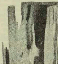
Section of a Greenhouse from Singapore destroyed by Termites.
