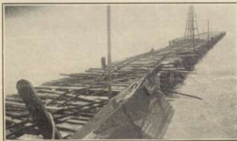
Levuka Wharf was badly smashed by the recent hurricane in Fiji. Heavy sea tipped the planking and rails.
